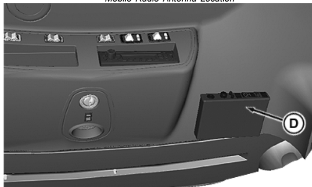
Mobile Radio Mounted In Right Rear Cab Corner
