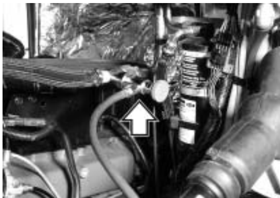
Recovery/Recharge Unit Area
