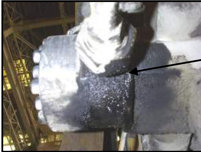
Fig. 63 High-pressure Fuel Leak at the Connector.
