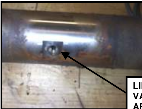
Fig. 48 USED AND CORRODED
