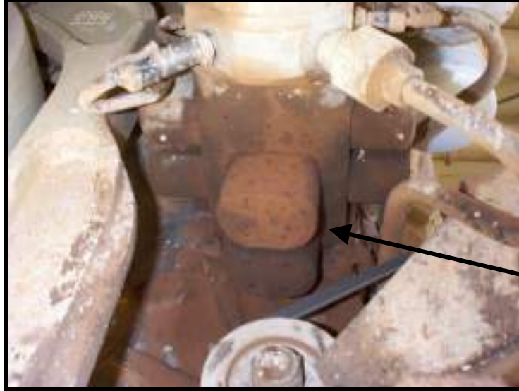
Fig. 21 High-pressure Fuel Pump Leak at Weep hole.
