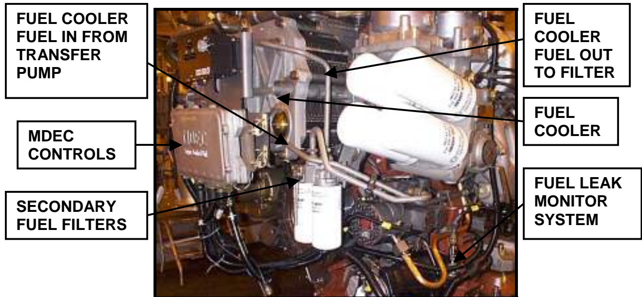
Fig. 93 Marine Fuel System (MDEC Controls)
