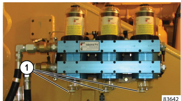
1. Water Drain Valves
