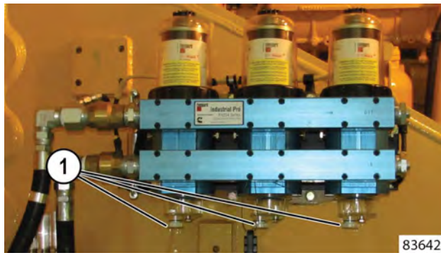
1. Water Drain Valves
