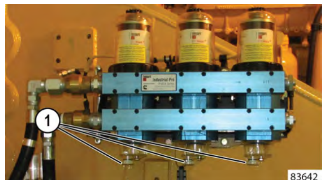
1. Water Drain Valves
