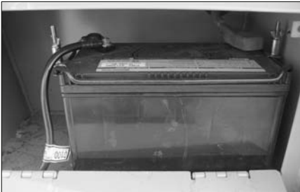
Typical Example LP Engine Truck
