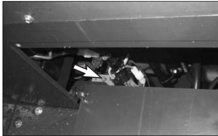
Typical Example LP Engine Truck
