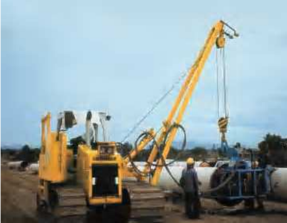
Pipefacing. The hydrostatic travel drive and the single joystick control allows exact placement of pipes.
