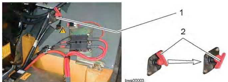
Turning off the battery main switch
