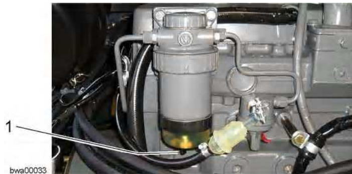
Draining off condensate
