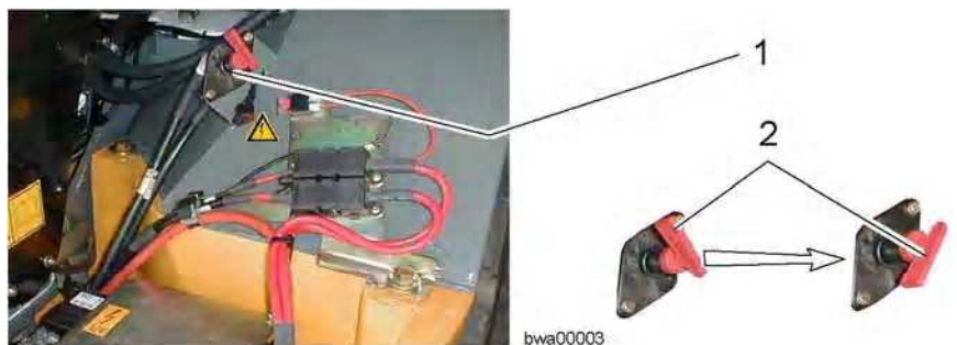
bwa00003 Turning off the battery main switch
