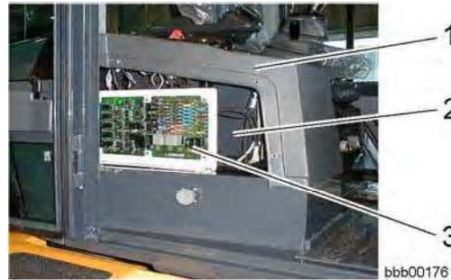
Fuse box with A4 control board
