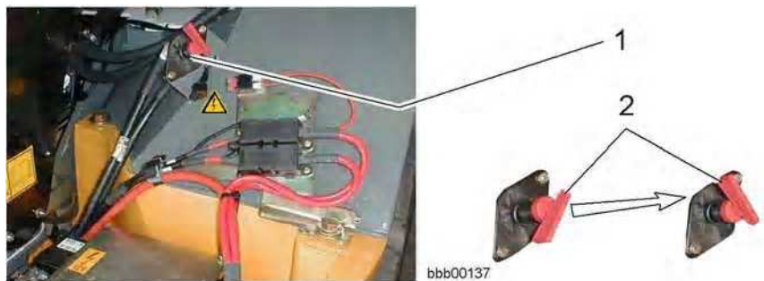
Battery main switch
