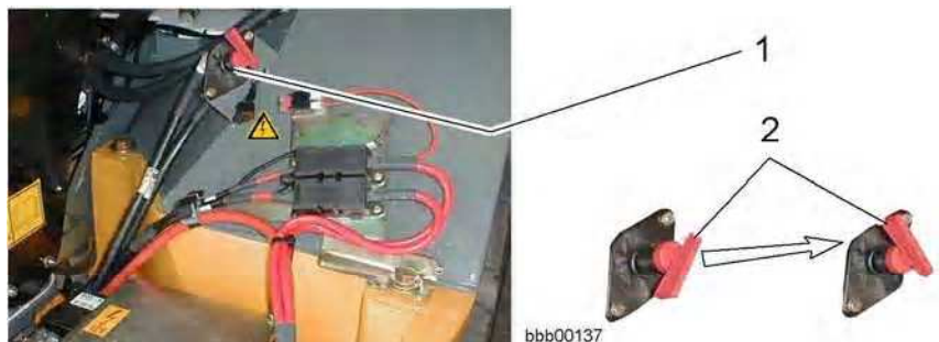
Battery main switch
