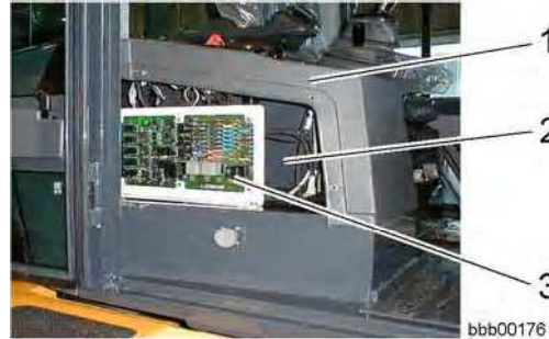
Fuse box with A4 control board
