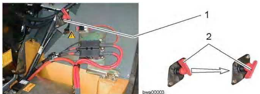
Turning off the battery main switch
