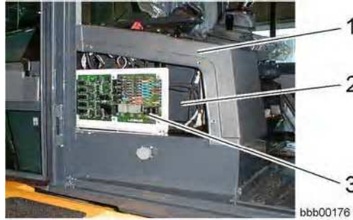
Fuse box with A4 control board
