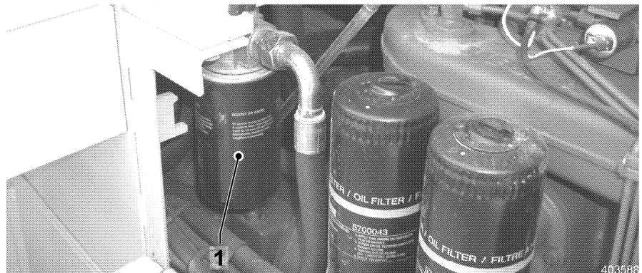
Replenishing oil filter
