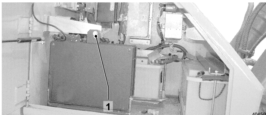
Central electric housing
