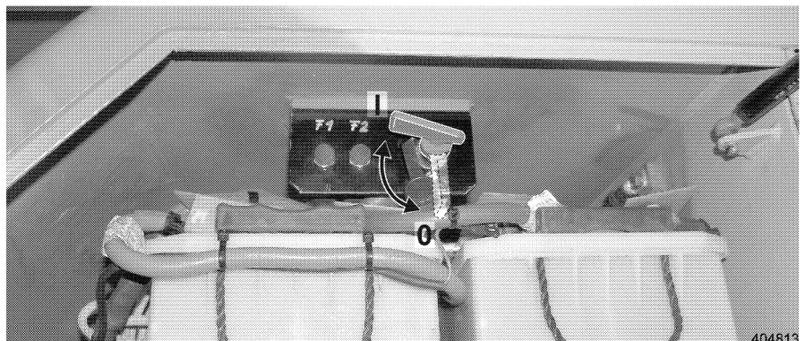
Battery master switch
