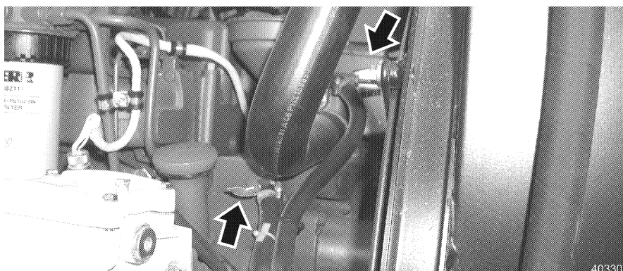
Shut off valves
