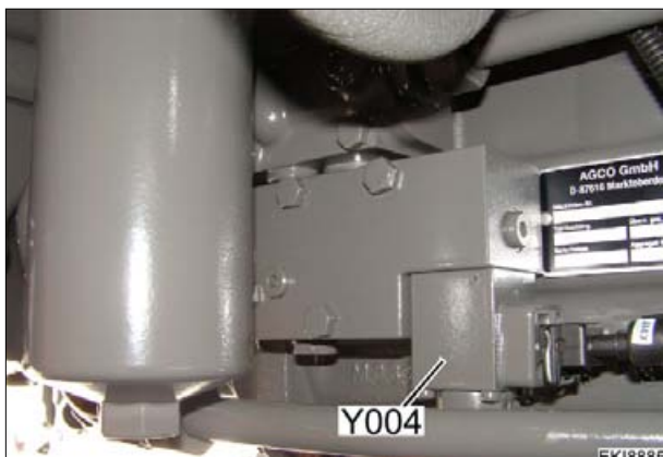
Y004 - solenoid valve (X317 - separation point)
