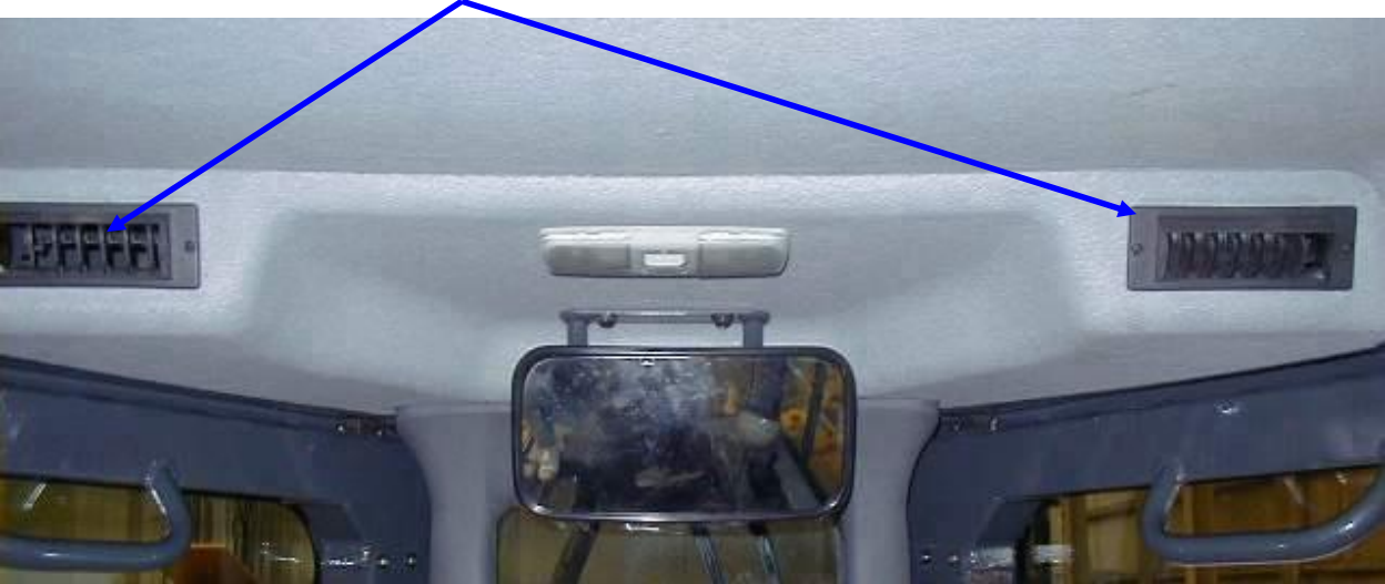
Air conditioner duct (At ceiling)
